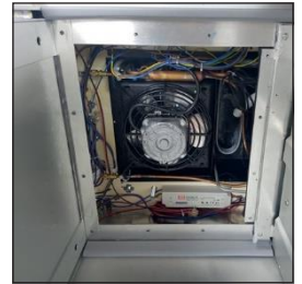
A5. Condenser compartment
